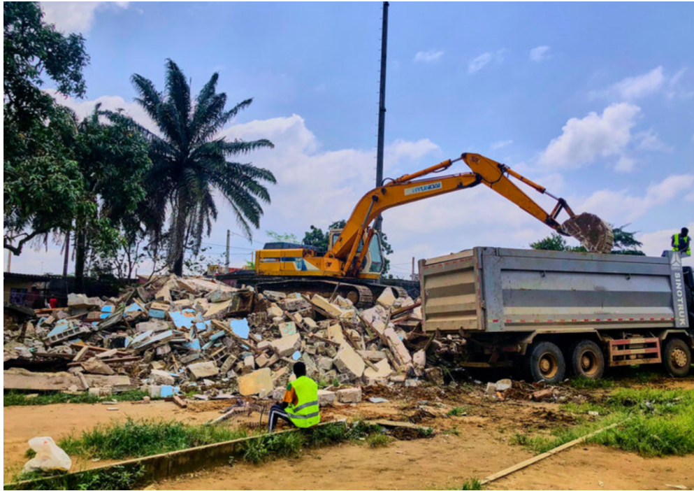
Demolition works for the creation of the Abidjan metro. Picture credit: Le Metro Abidjan .
